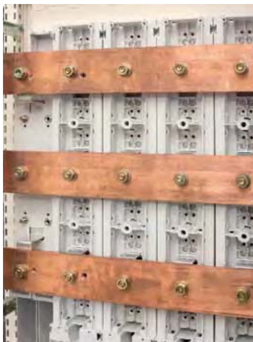
ISFL250 (direct connection on 185 mm 2 busbar).
