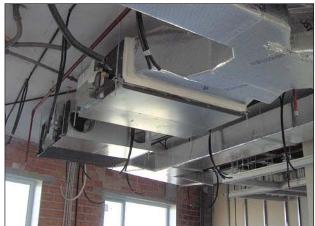
Lossnay units are suspended from ceiling.
