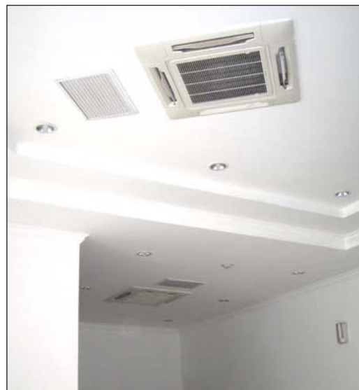
Cassette-type indoor unit installed in the ceiling.
