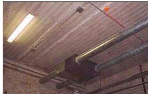
Lossnay unit is suspended from ceiling.
