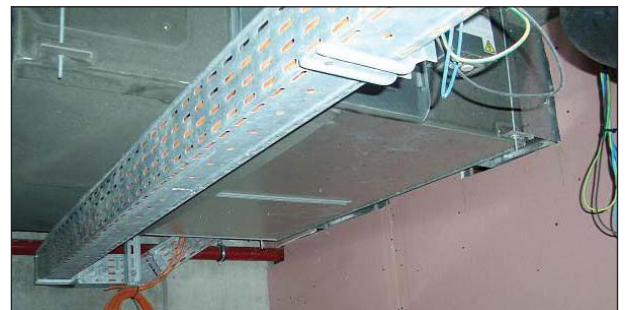
Lossnay unit is suspended from ceiling.
