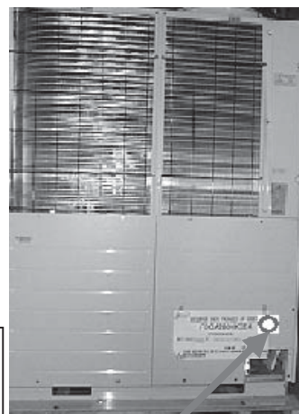
Fig. 6.11 Operation valve Open marking
